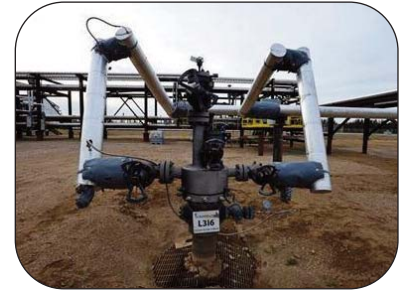
Steam Injection Well
