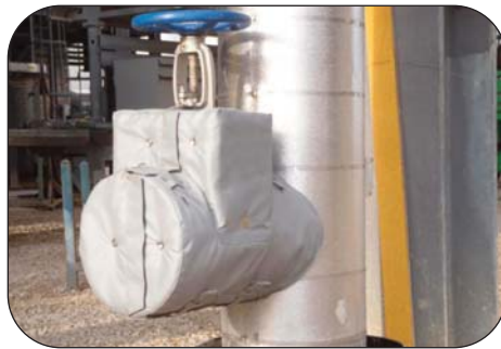
Valves and Equipment
