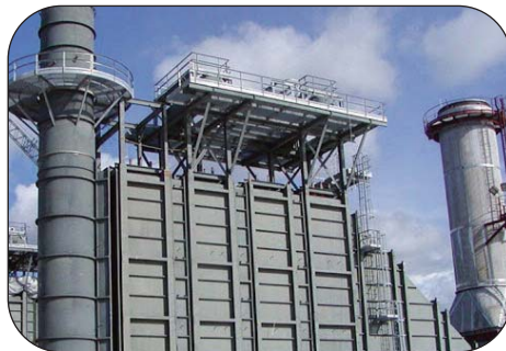
Clean Combined Cycle Power Generation
