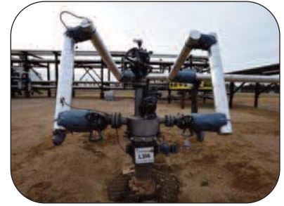
Steam Injection Well
