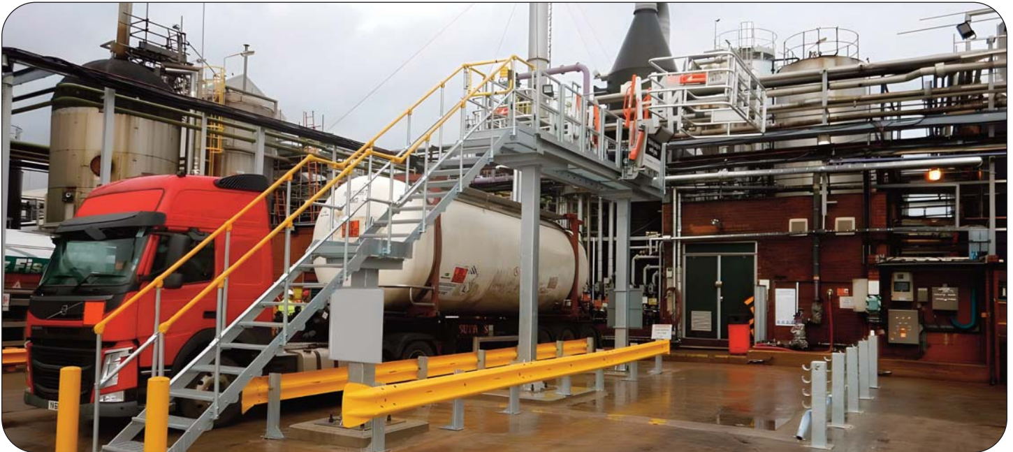
Chlorine Unloading Station
