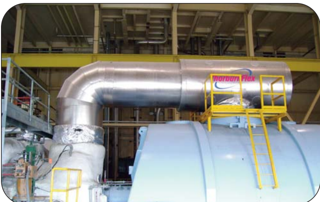
Thorburn crossover expansion joint in service on a steam generator
