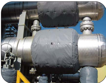
Process piping and equipment left without a properly designed thermal insulation cover can freeze and fail to properly operate.
