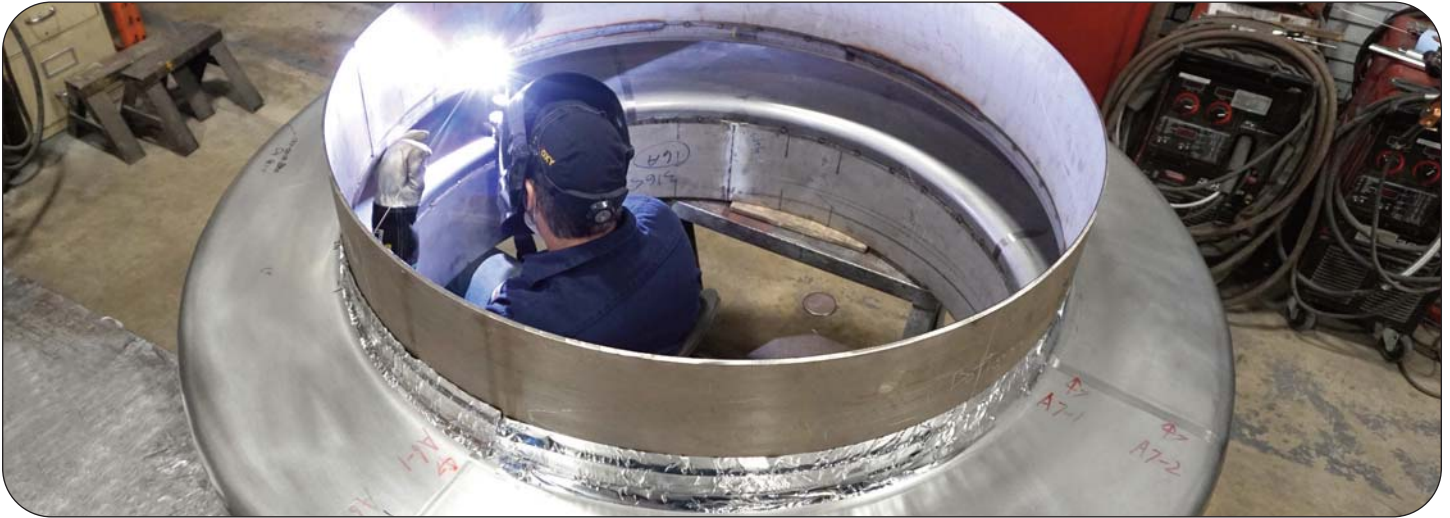
Welding a Thorburn Series AFU Inconel 625 250mm height single convolution bellows expansion joint without crest weld
