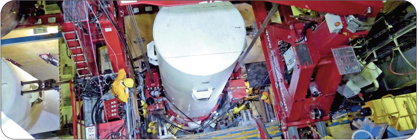
Steam generator at Embalse power plant
