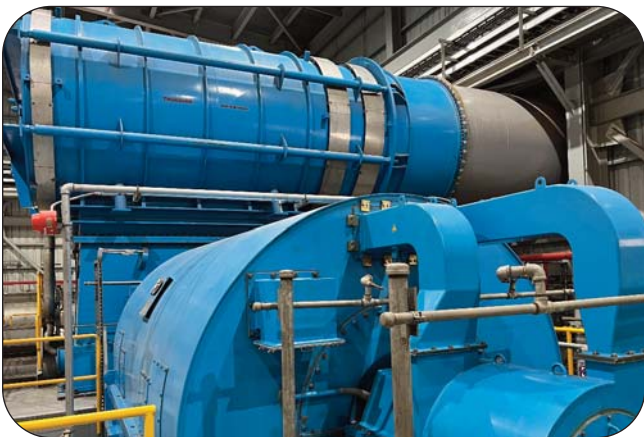
Thorburn's crossover expansion joint installed on a geothermal power plant
