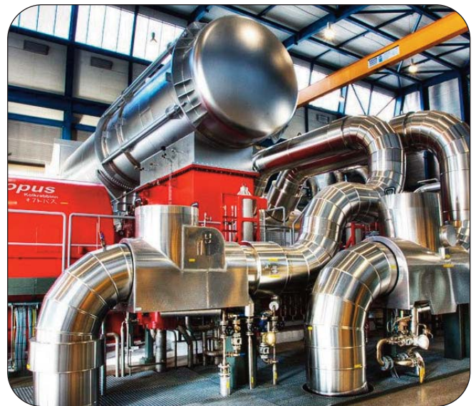
Steam generator with a crossover expansion joint in a geothermal power plant
