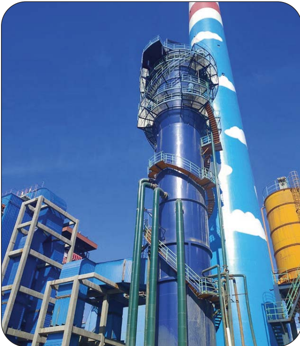
Circulating Fluidized Bed (CFB) Power Plant
