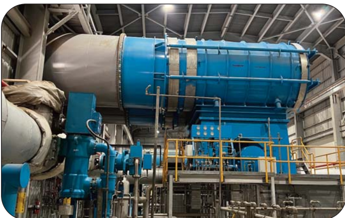
Thorburn PBEU universal elbow pressure balanced expansion joint for a steam turbine in a geothermal power plant near Leon, Nicaragua, Central America
