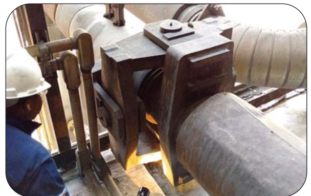
Thorburn Single Flex™ Series GF gimbal type expansion joint installed in a high pressure steam piping system
