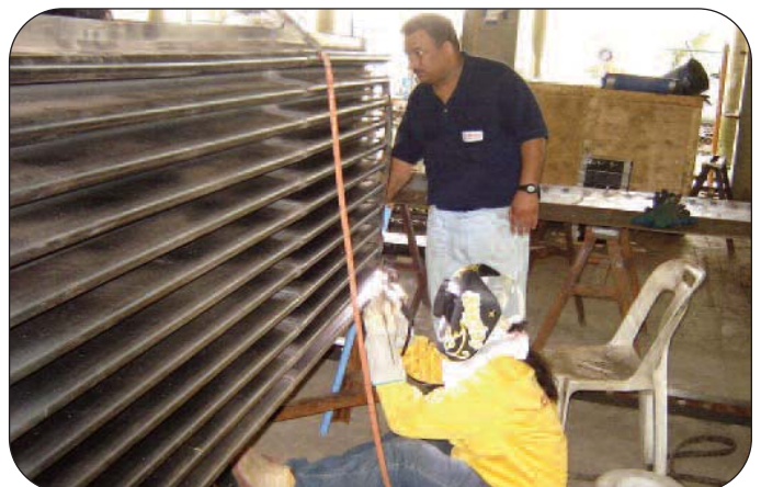
Thorburn's Malaysian team welding a Duct Flex™ expansion joint for the Tanjung Bin power station in Johor Pontian Malaysia
