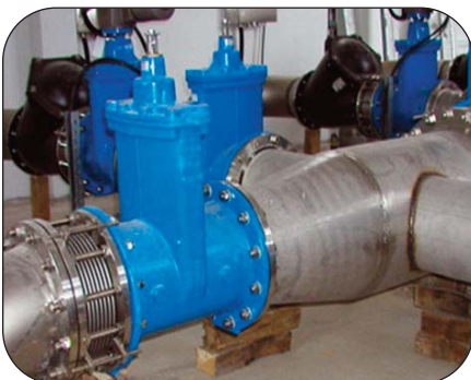
Single Flex™ bellows with control rods installed on a pumping station
