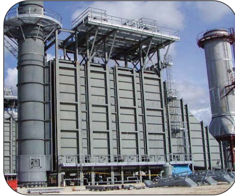
Clean Combined Cycle Power Generation
