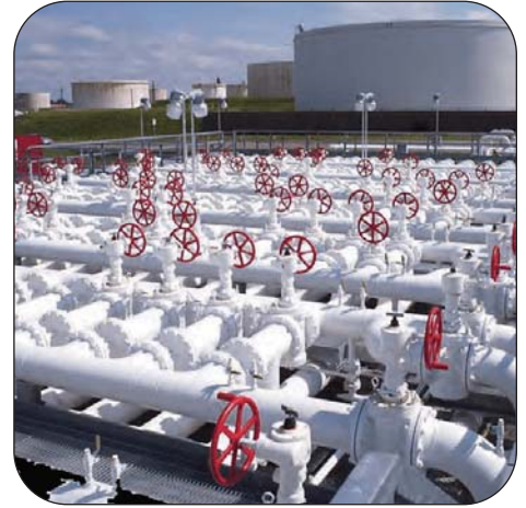
Storage Tank Seal Valves
