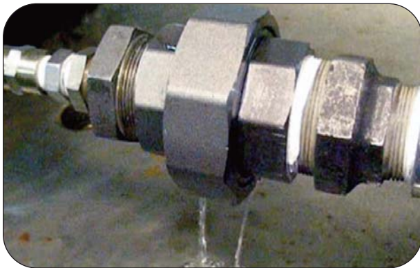
3000 lb MSS SP83 forged union with rusted sealing surfaces leaking with no pressure in the piping line. Once the sealing surfaces are rusted or compromised, they will always leak no matter how much torqued is applied
