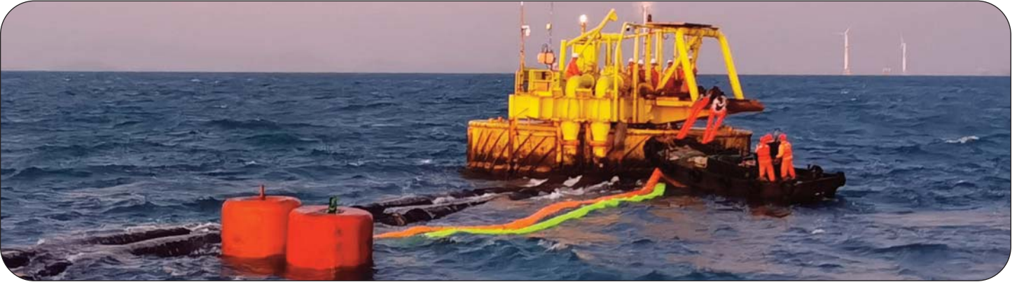
CBM/MBM Cargo Transfer System with Submarine Hoses
