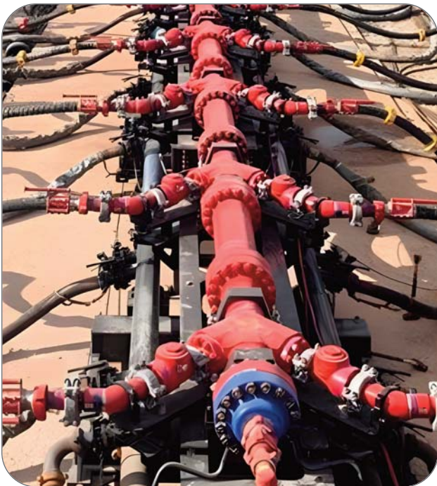
Fracking hoses connected to tank manifold
