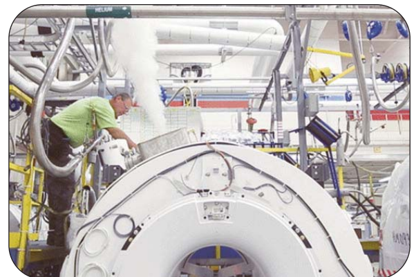
Thorburn's Met-O-Seal Series MTS4 hose coupling used for loading liquid helium in an MRI machine at -269°C (-452°F) just above absolute zero. Magnets at that temperature lose all electrical resistance and become superconducting thus produce the same magnetic field for a thousand years with no more power required.
