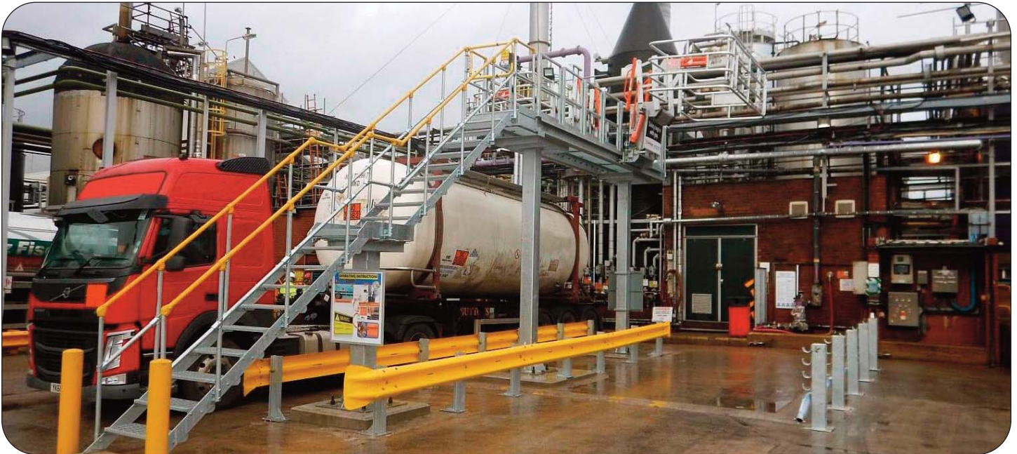
Chlorine Unloading Station
