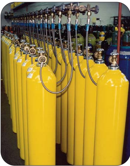
Pigtail hoses on gas cylinder manifold
