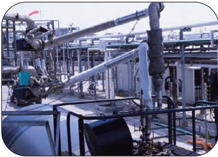
Freeze protected chemical loading/unloading
