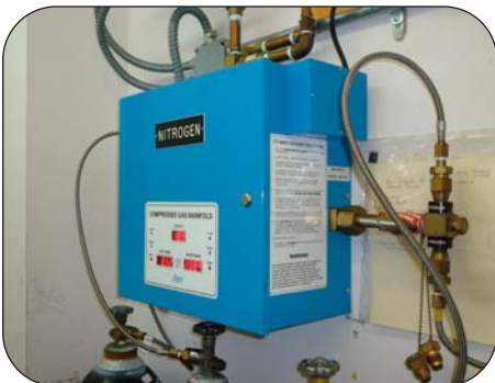
Pigtail hoses on nitrogen gas manifold
