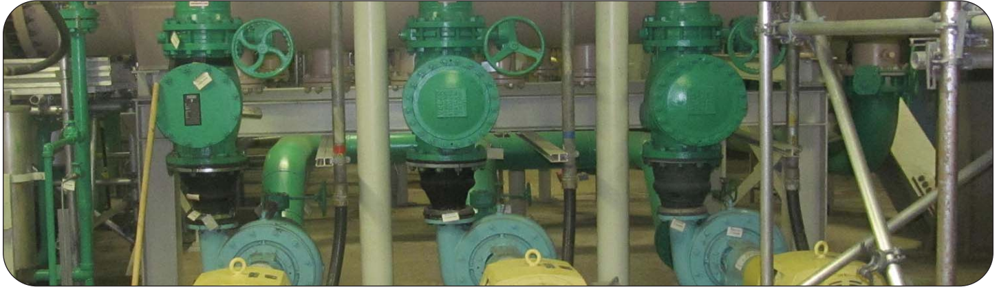
Thorburn's 42HP-CR Concentric & 42HP-OR reducing expansion joints installed in pumping station at the OPG Pickering nuclear reactor
