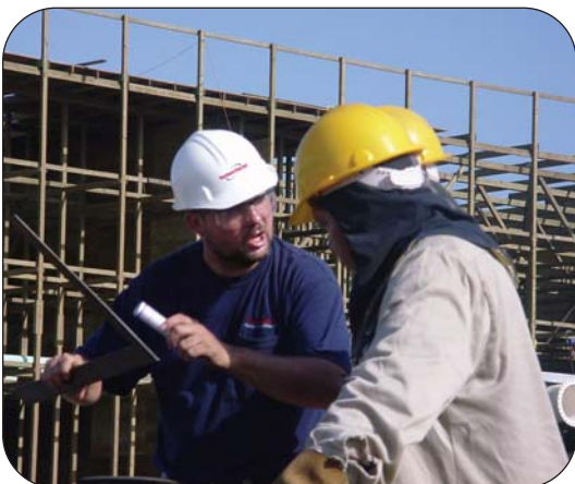
Thorburn's site team instructing a technician on how to properly install Thorburn's Mighty Spool pressure piping expansion joints
