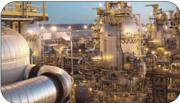
Thorburn was awarded the contract for the Syncrude Fort Hills, Canada high pressure slurry rubber piping expansion joints
