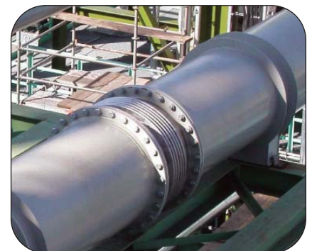
Hot-flex installed in a sulphuric acid transfer line
