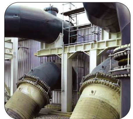
Thorburn rubber dismantling joints installed in an FRP piping system
