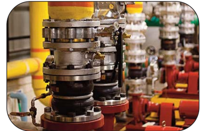
Thorburn model 201 twin sphere joints installed at a pumping station
