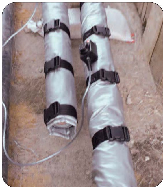
Thorburn's ThermaCover™ Series TCT-HT removable insulation jacket with integral heat tracing elements
