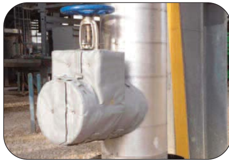
Valves and Equipment
