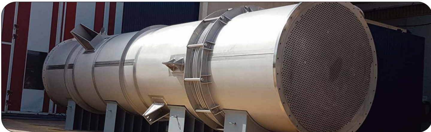
Thorburn Series SF Single Flex tied bellows installed on a heat exchanger
