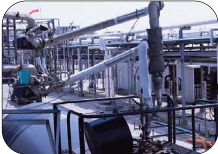
Freeze protected chemical loading/unloading
