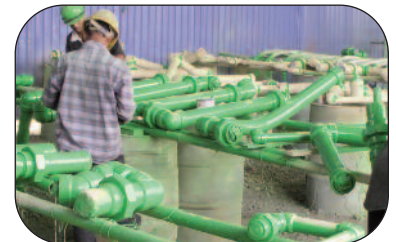
Rigid Piping Systems with Full Blasting & Painting Capabilities
