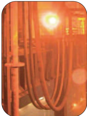
Installed Oxygen Lance Hose Assemblies
