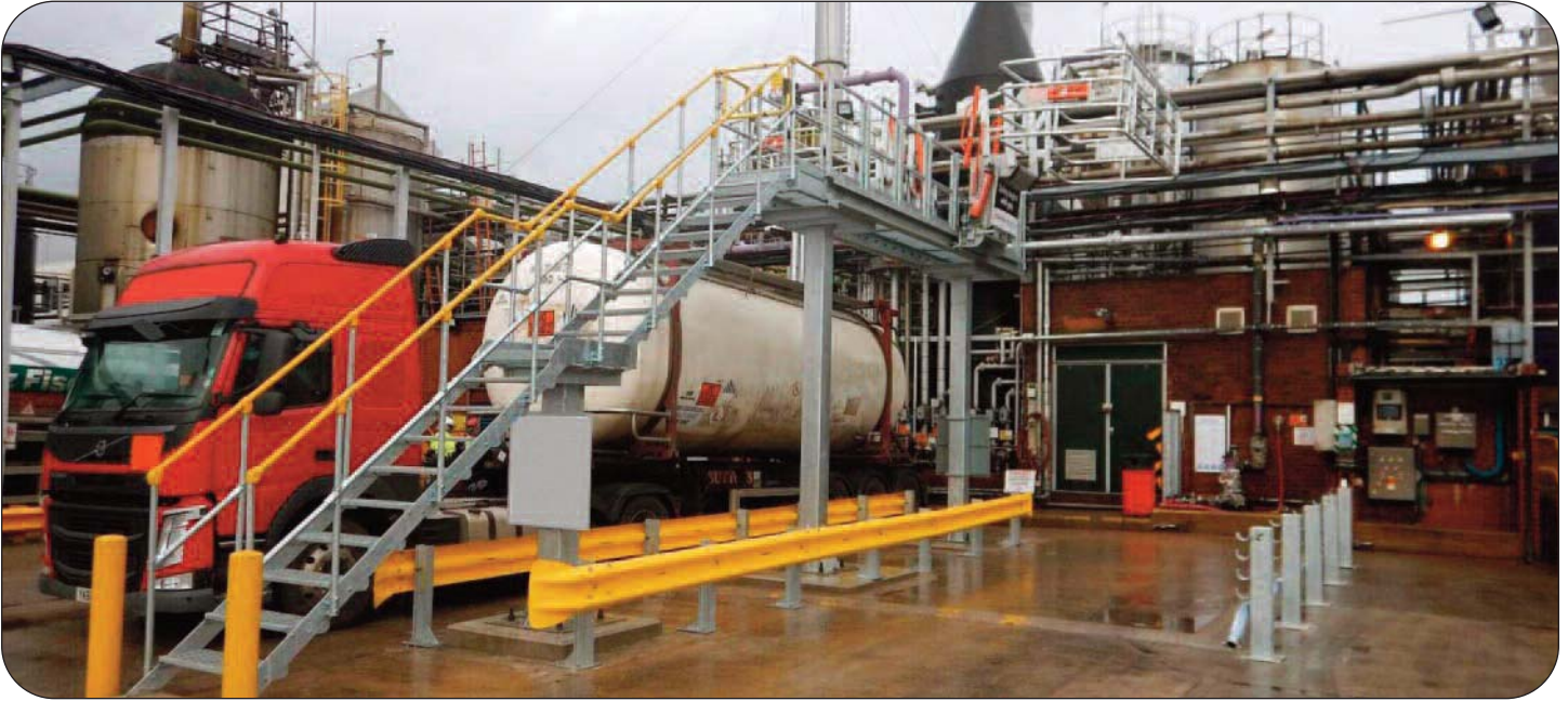
Chlorine Unloading Station
