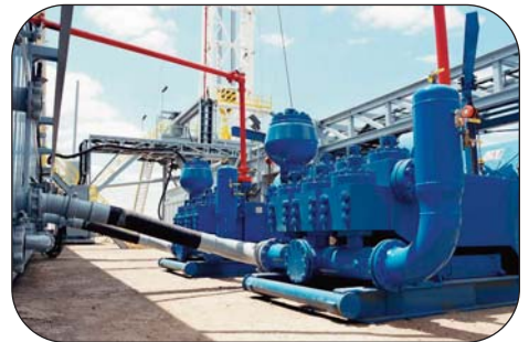
Mud Pump Discharge Lines
