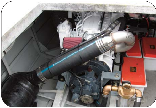
Wet exhaust system with hardwall hose
