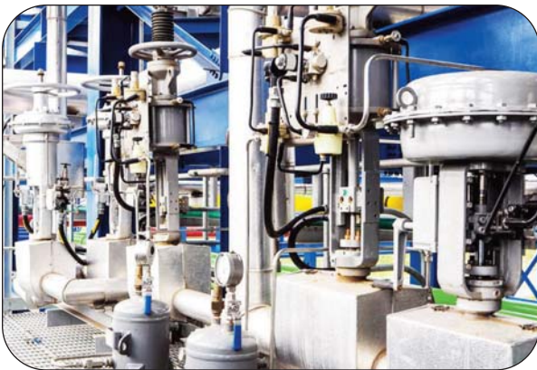
Condensate recovery system
