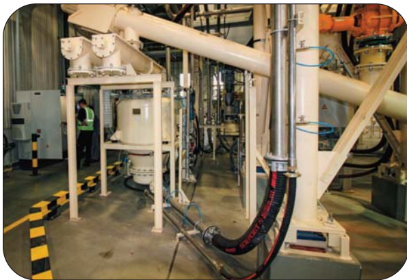
Pneumatic Conveying System
