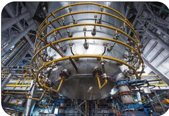
Pulverized Coal Injection (PCI) System
