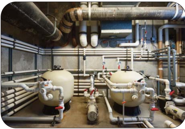
Commercial pool plumbing
