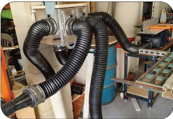
Woodshop sawdust collection system
