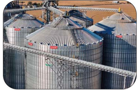
Silo Grain Conveying Systems
