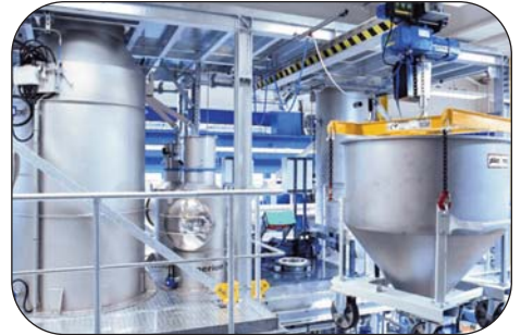
Pneumatic Conveying System
