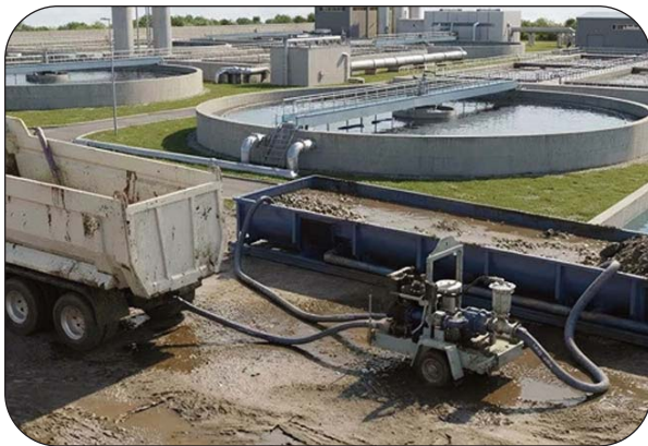
Slurry mixing and transfer pump
