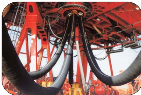
Oil Rig Fluid Handling
