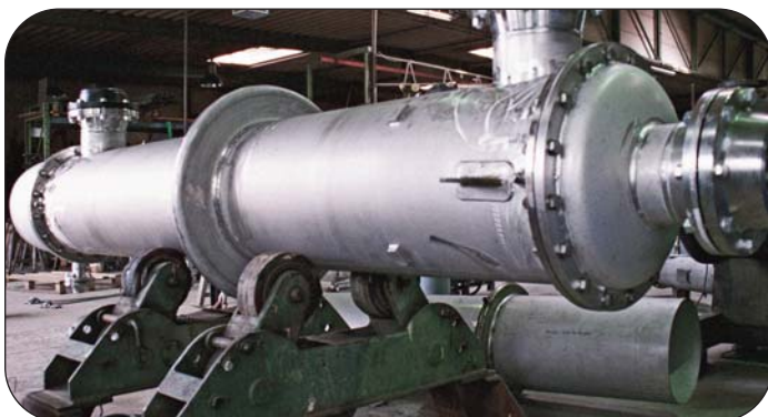
Thorburn lens bellows installed on a heat exchanger
